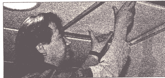
David removes a panel of the drop ceiling to check out the insulation upgrade
